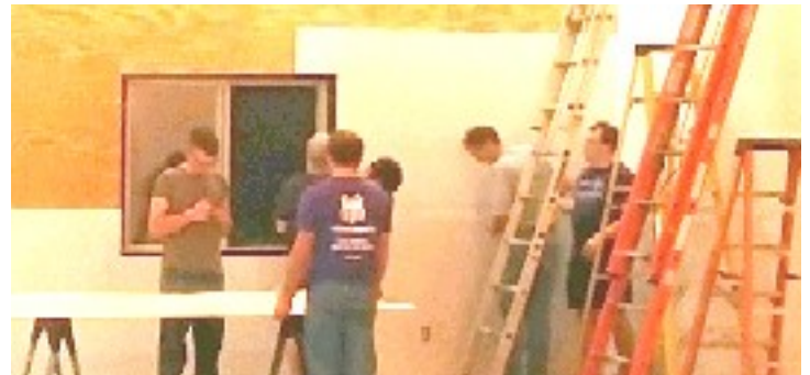
Men in the church (Nate 2 nd from right) hanging drywall to improve our rented church meeting place.
